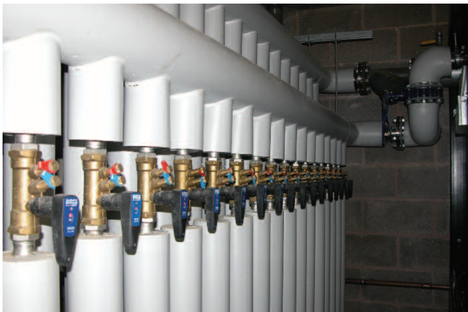
Heating pipework and connections are insulated to a high level
